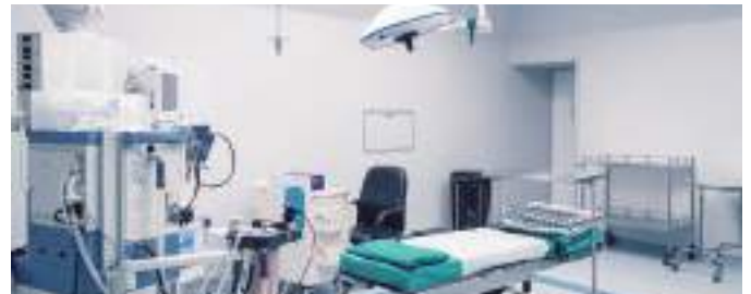
Medical Equipment Monitoring
